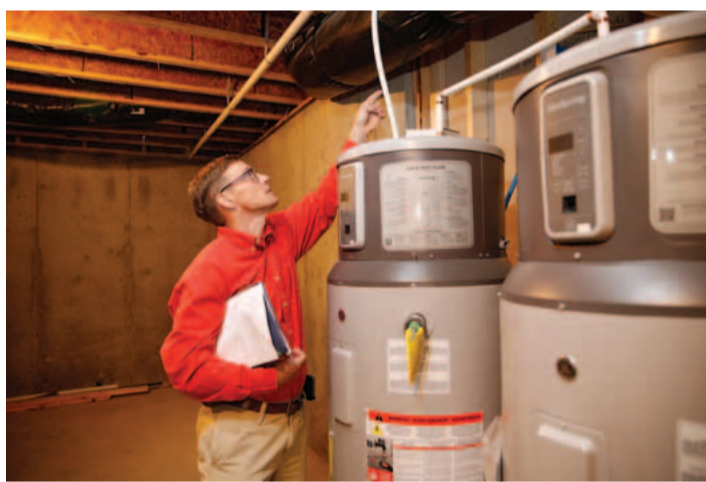
Jeff Hall of J. Hall Homes explains the routing system that brings hot water to any faucet in the home in just seconds.
